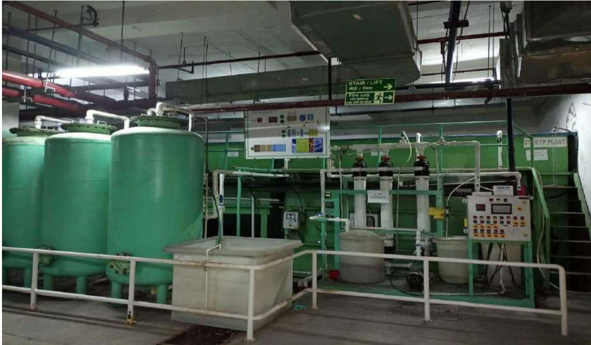
Figure 5. Effluent Treatment Plant
