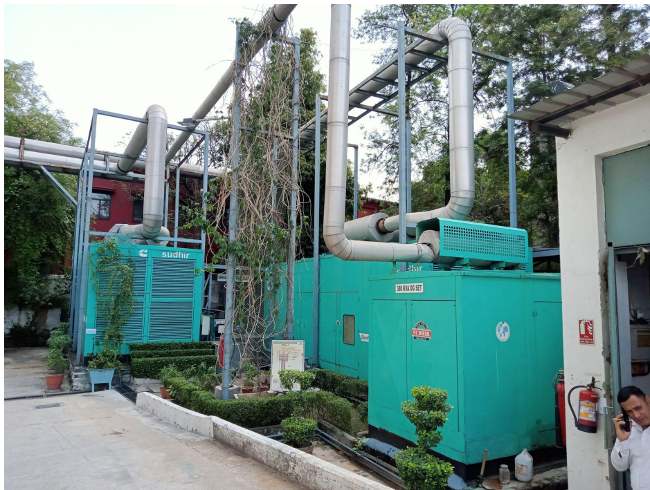
PHOTOGRAPH OF DG SET STACK/DG SET
