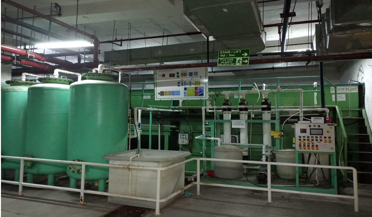
PHOTOGRAPH OF SEWAGE TREATMENT PLANT 70 KLD at A Block and 120 KLD at B Block/OR RELATED COMPONENTS
